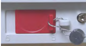
Locked with Wire Seal
